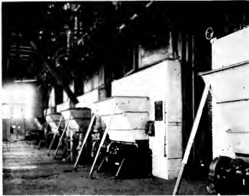
Tending Floor of Boiler House. Travelling Weighing Hopper Charging No. 3 Stoker.
